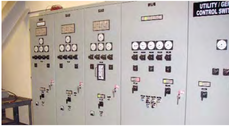
Figure 4. This photo depicts a closed transition utility and generator paralleling switchgear control panel. The system can incorporate up to two medium voltage utility feeders and several medium voltage large kW generators. The paralleling gear also contains all control functions including system load analysis, generator starting, generator shedding based on actual load, generator use rotation, load shed if more than the redundant generator fails as well as other control functions.
