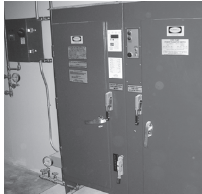
A fire pump controller should be separated from the main service and the generator to protect it from a potential fire at those points.
