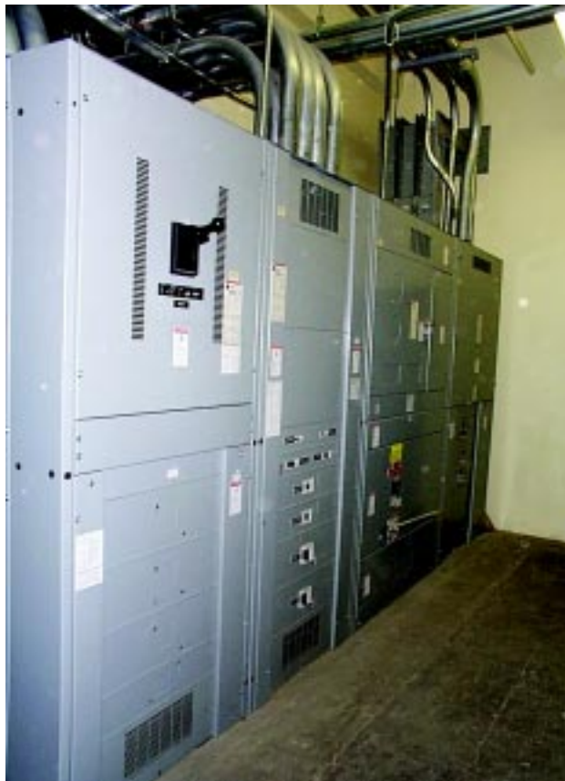
This 4,000A service switchgear requires AIC bracing and overcurrent protection in excess of 65,000AIC.
