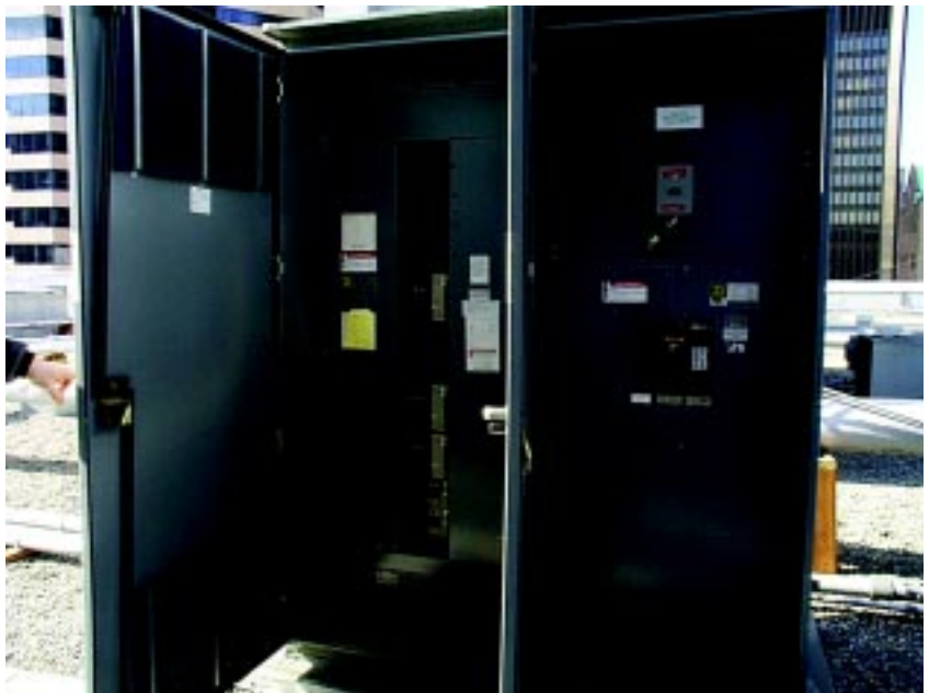
AIC calculations for this roof-mounted distribution panel must include motor contribution factor.
