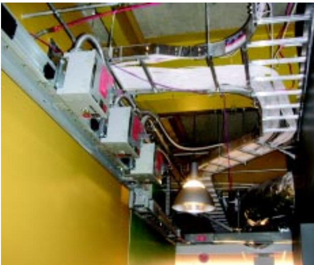
Photo 3. Plug-in style 1,200A busway and cable tray allowed for greater flexibility for future remodeling projects.
