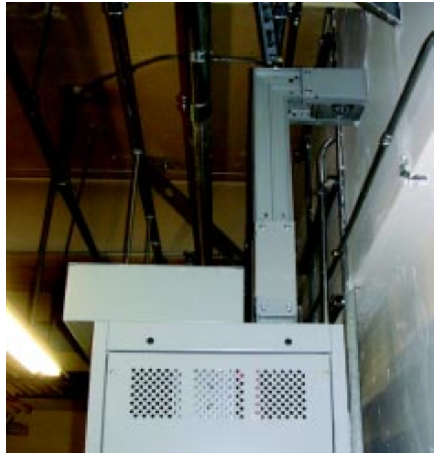
Photo 2. Pipe and wire from the transformers led to a 1,200A disconnect, shown here from the side to reveal the transition to 1,200A busway.
