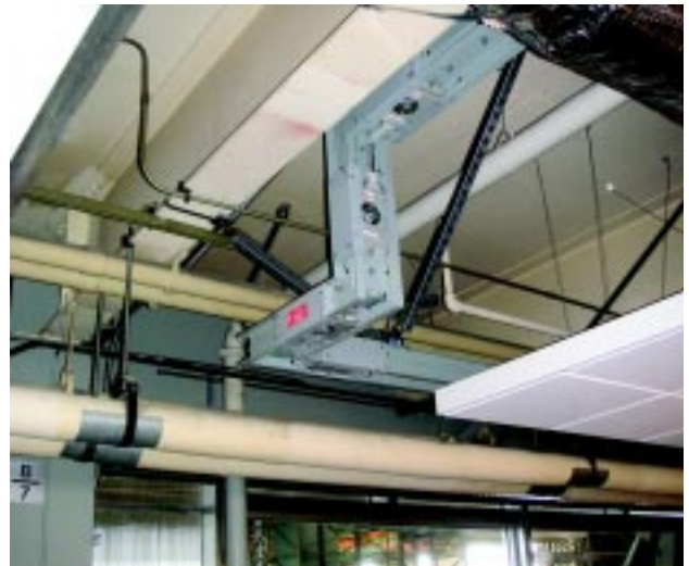
Photo 4. The plug-in style distribution also made it easier to maneuver around obstacles like these drop clouds (suspended panels at right).
