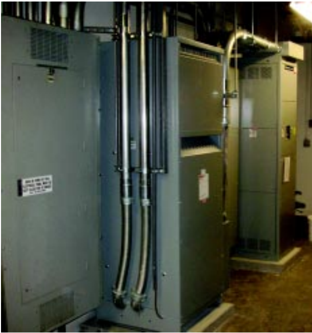
Photo 1. Using harmonics-mitigating 300kVA transformers with 1,200A busway proved to be the most cost effective solution.
