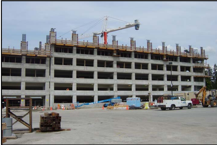
Typical parking structure that would require roof parking egress lighting to be fed from an emergency electrical system under the provisions of the IBC.
